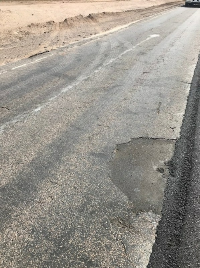
Existing Condition/ some patching
