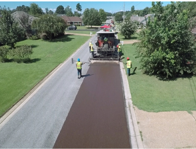
Chip Seal and Microsurfacing was applied to this neighborhood in Rankin County
