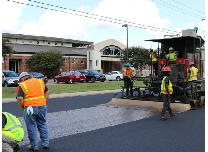
Scrub seal and premium micro surfacing was applied to this high traffic road in Rankin County.
