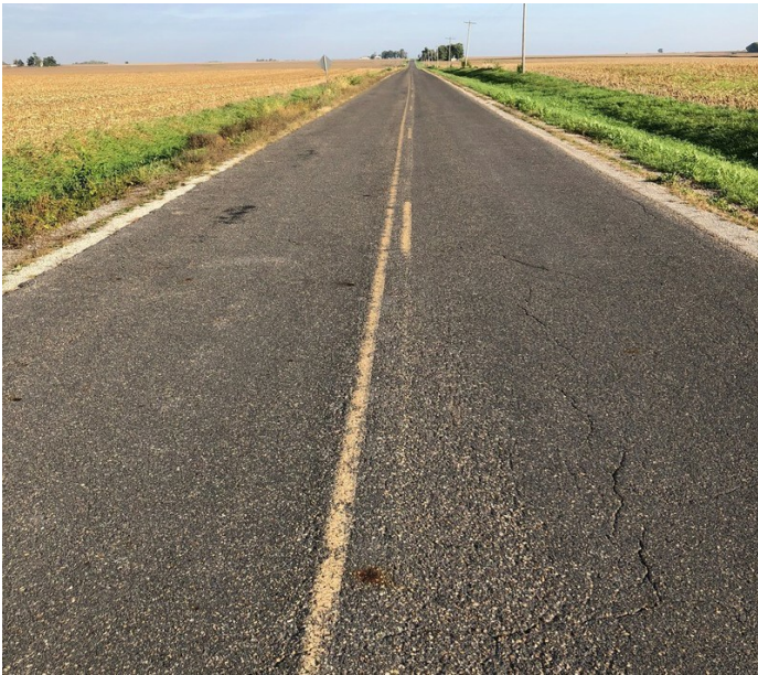
Original Narrow, Distressed Pavement
