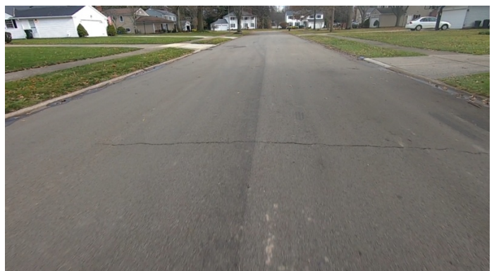
Upcoming Crack Seal Candidate
