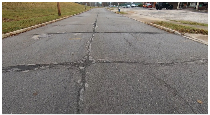
Roadway that Did NOT Receive a Crack Seal Treatment at the Right Time
