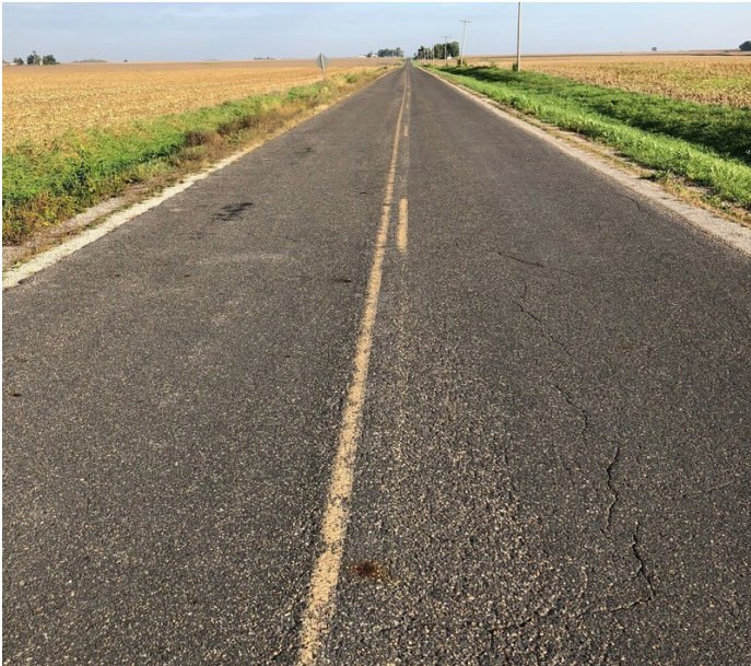
Original Narrow, Distressed Pavement
