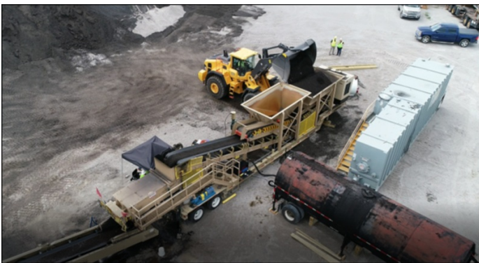
The nearby cold central plant being fed with RAP from the stockpile
