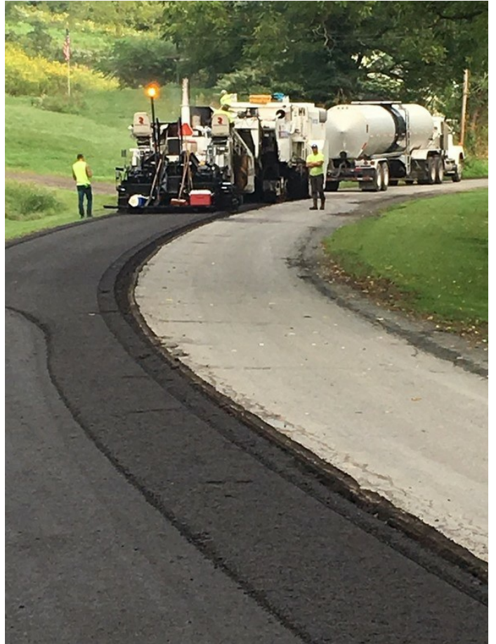
Cold-In-Place Recycling "train" with tanker of CSS1-h emulsion hooked onto milling machine and paver.
