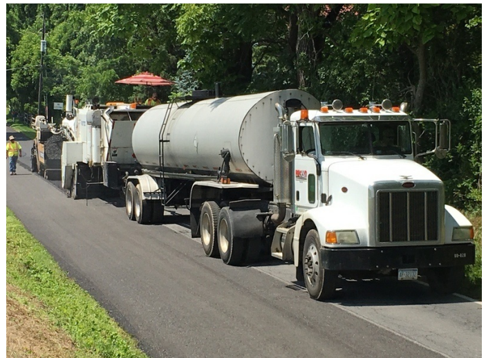
Cold-In-Place Recycling "train" with tanker of CSS1-h emulsion hooked onto milling machine.
