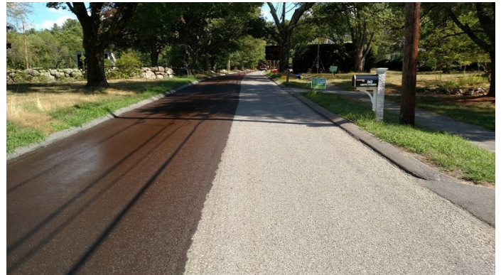
Micro surfacing over chipseal on one side and chipseal on other side of roadway
