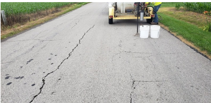
Existing Pavement Condition along Jackson Road, cracking throughout the project included longitudinal and block cracking
